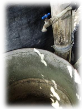
Water connection of previous system. Faucet was found open, but had been without water for eight days.
