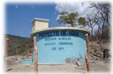
Finished storage tank in Guaricayán
