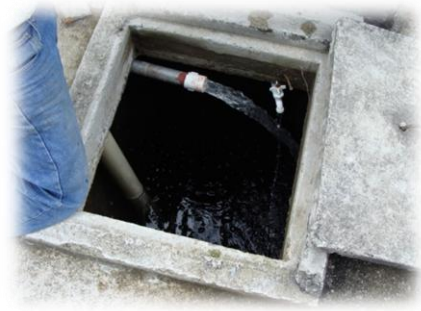
38 GPM entering tank through new conduction line
