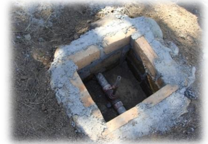
One of four air valves with valve box
