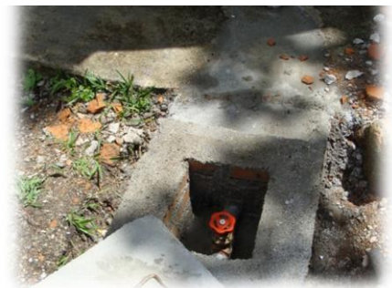
Inlet valve to storage tank with valve box
