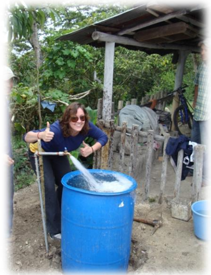
Water connection turned on for the first time at house in El Zurzular
