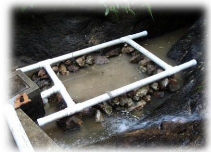
Finished, installed filter
